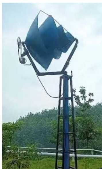
Fig. 2. Wind energy installed in the tourist village
