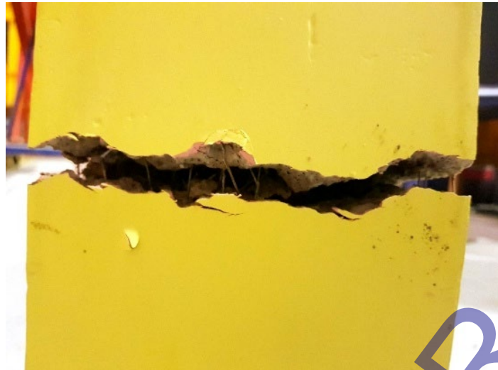
Fig. 6. Crack in concrete beam reinforced with steel fibers 50 kg/m 3 . Source: Authors.
